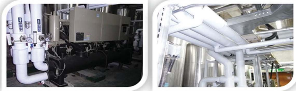
Figure 2.0 Hot Water Produced from Heat Pump System
