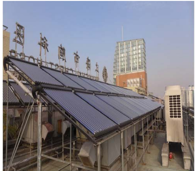
Picture 3: solar collectors on the roof
