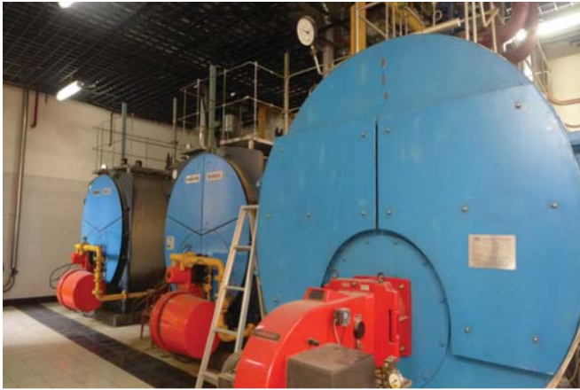
Picture 1: The boiler room after transformation
