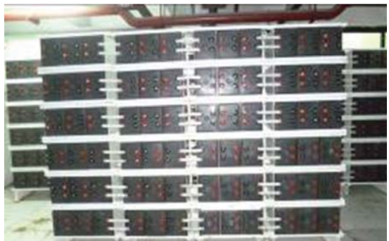
Figure 6. Battery bank for solar energy
