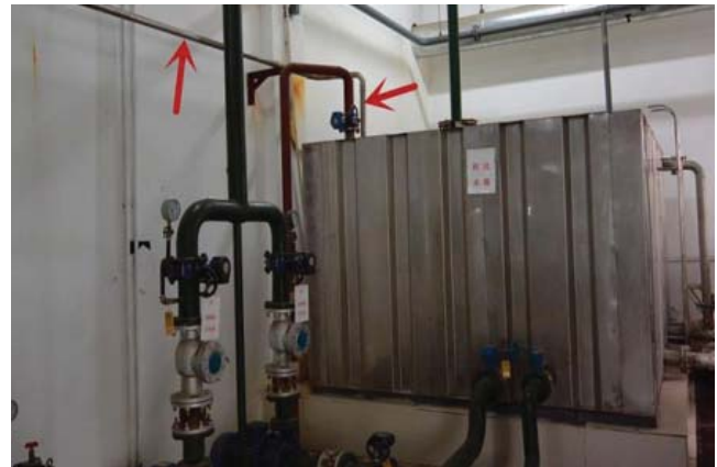
Picture 3. Soft water transfers to the water tank in boiler room
