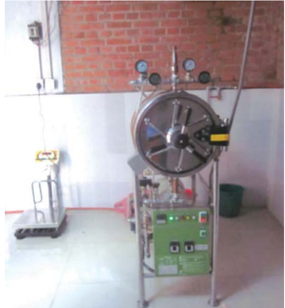
Figure 8. Autoclave used for treatment of infectious waste
