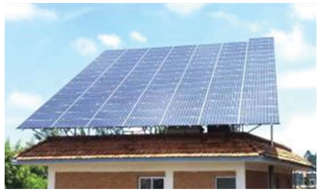
Figure 4. Solar panels at the roof top of the hospital
